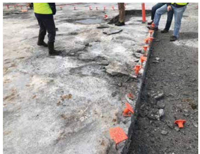
Fig. 3: Surface damage (spalling) of the podium level due to fire
